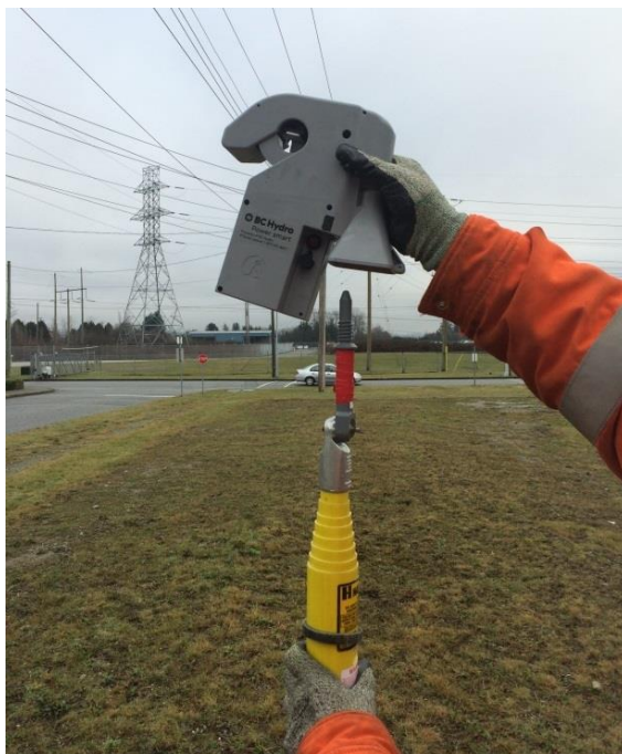
Photo 1: TGI Raptor meter used by B.C. Hydro to balance energy flows
